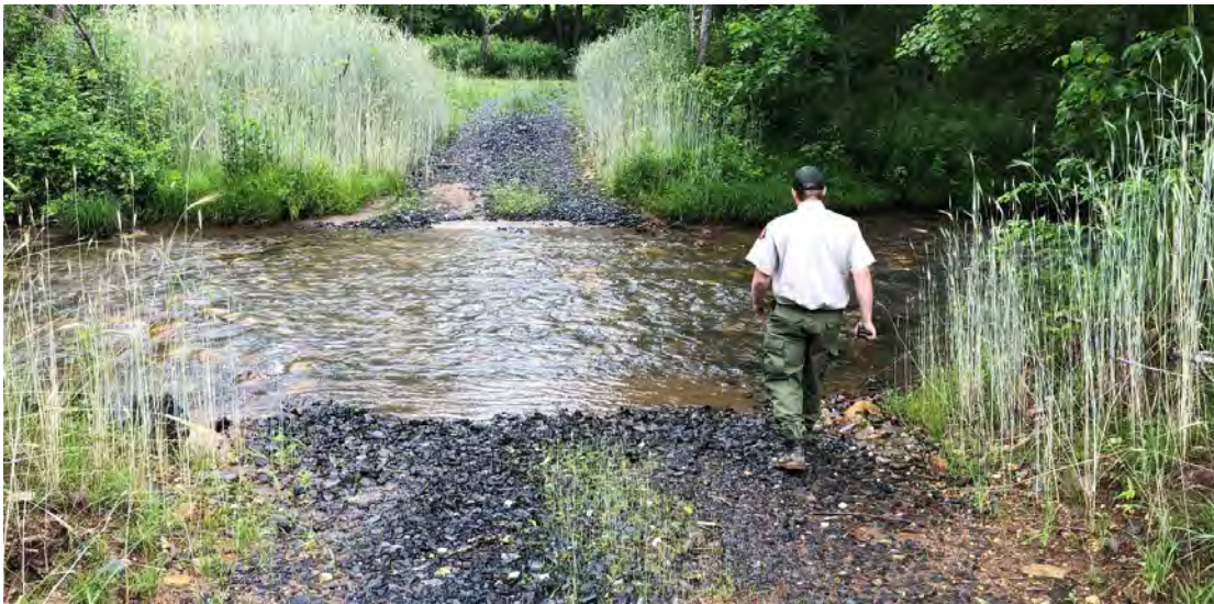
Figure 6N: A well-stabilized ford crossing with gentle road approaches Photo note: This ford crossing has ample stabilization on the roads and along the berms. The gentle approach grades help make this an ideal location for a ford.
