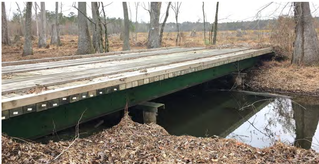
Figure 6A: Permanent bridge stream crossing for forestland access
