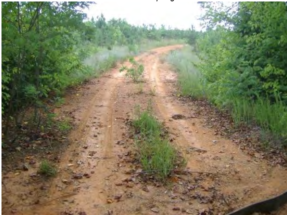
Figure 7C A forest haul road with lower road standards than figure 7B Picture note: Compared to 7B, this road is narrower, has more bare soil, and fewer water control structures. However, the traffic volume is much less and therefore may not need as many BMPs to provide similar water quality protection as the road in figure 7B.
