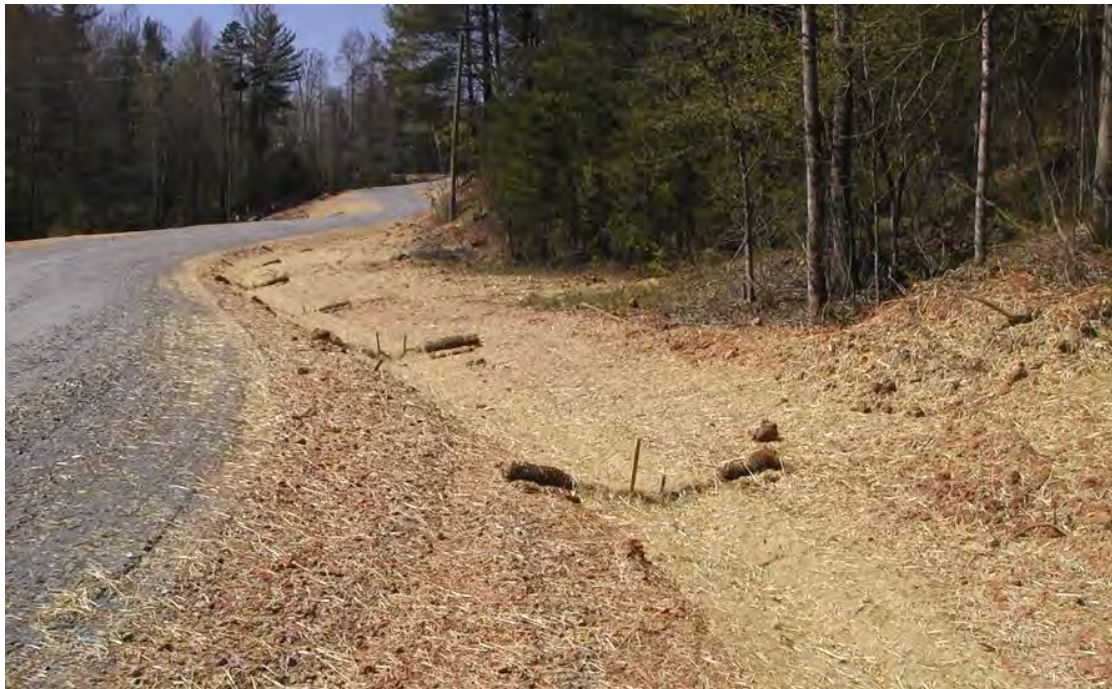
Figure 5X: A series of coir fiber check dams and straw matting along a graveled road Picture note: Blankets must be firmly secured to the soil with wire metal staples to prevent runoff from up-lifting the blanket and washing underneath.
