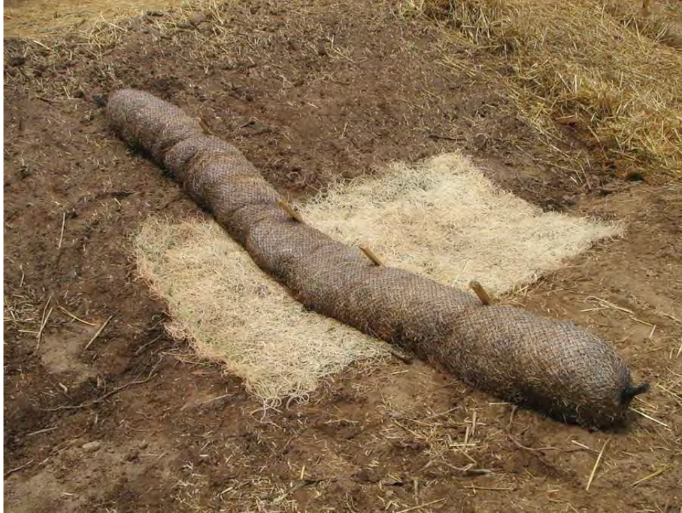
Figure 5W: Check dam made with a coir fiber wattle log, on top of excelsior matting Picture note: Wooden stakes are used on either side, not punctured through the wattle log.
