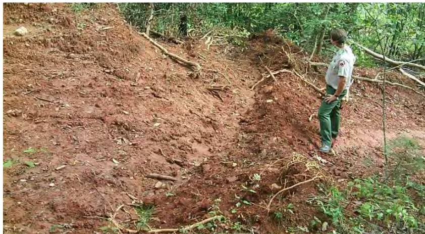
Figure 5D: View of the trench along the uphill face of the same waterbar
