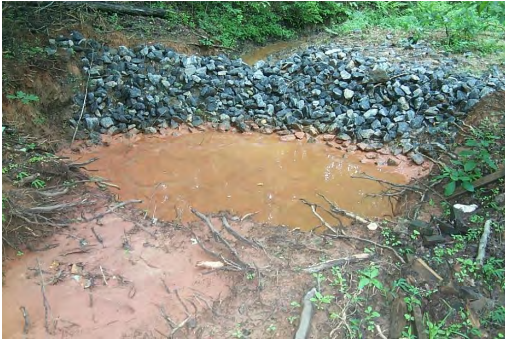
Figure 5N: A functioning sediment pit excavated alongside a forest road Picture note: This sediment pit is located in a good position to capture sediment that flows off this graveled, outsloped road. The pit is positioned away from the stream (in background).
