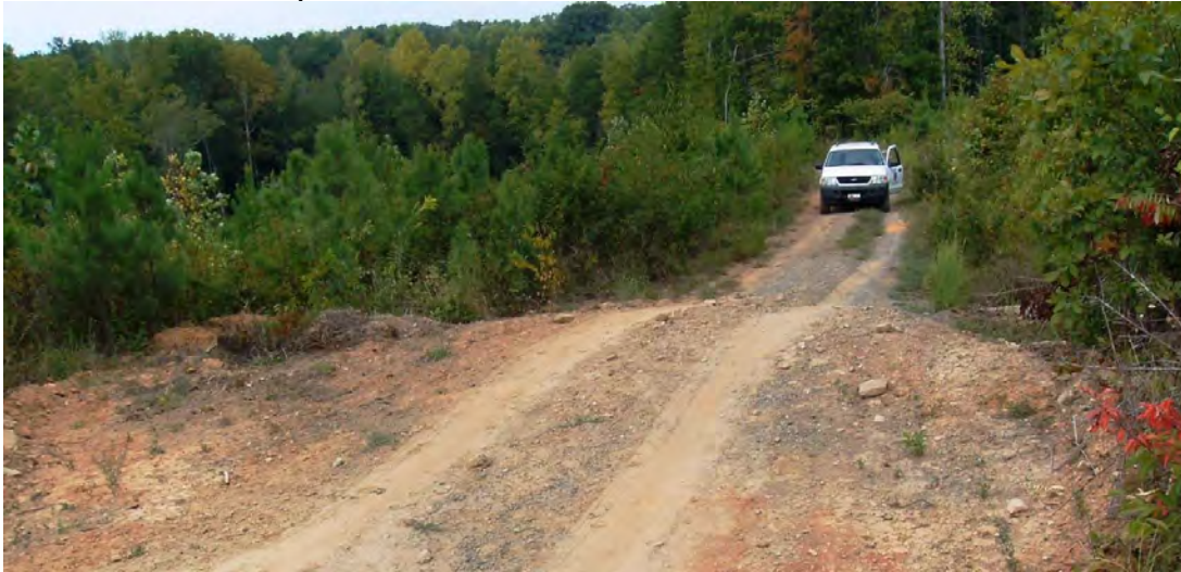
Figure 5E: A rolling dip on a forest haul road
