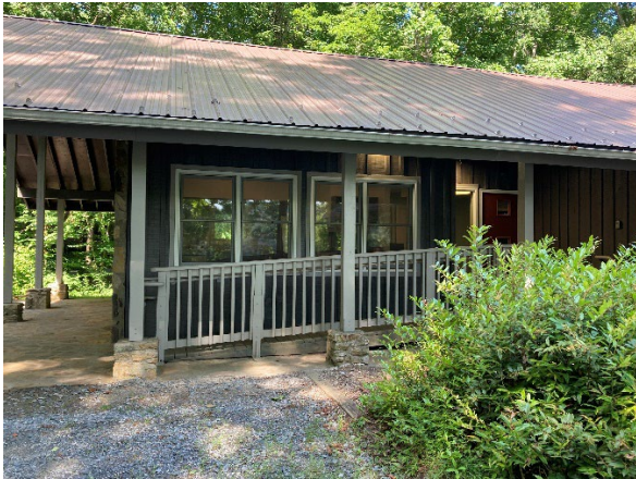
The renovated exterior includes a covered ADA compliant ramped entry into the building.
