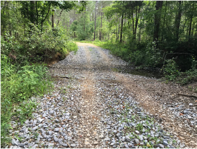
Figure 8. Ford stream crossing. Correct: Use of rock on stream crossing approaches and stream bottom.
