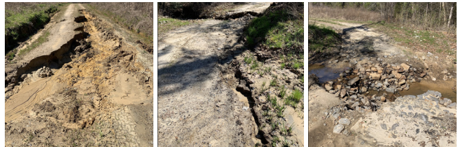
Figure 6. Permanent forest road culvert. Incorrect: Severe erosion on forest road stream crossing approach with erosion leading directly into the stream. This resulted in three issues: (1) water quality degradation from sedimentation, (2) washed out culvert, and (3) the need for significant road and culvert repair. No water diversion device or rock was applied on the stream crossing approach.
