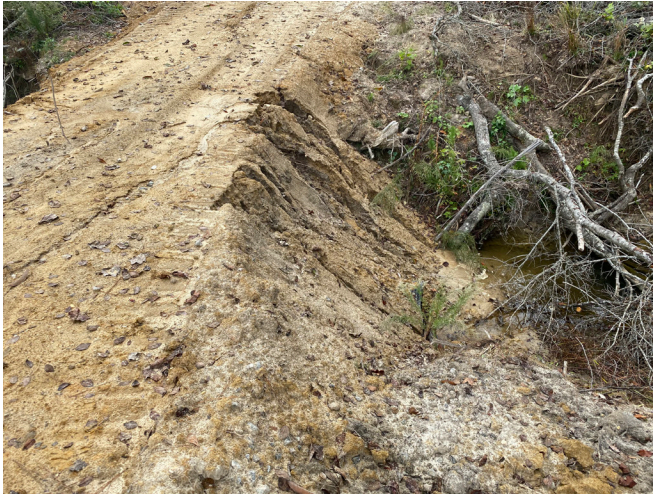
Figure 11. Temporary culvert stream crossing. Incorrect: Culvert diameter is too small for the width and depth of the stream and is not extending out long enough on both sides. The fill material is too steep and unstable, leading to sedimentation issues.
