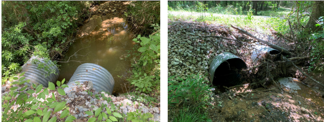
Figure 3. Permanent forest road culvert. Incorrect: Outflow side (left) is not on the stream channel bottom that is not allowing passage of fish and aquatic organisms and is also creating a plunge pool. The inflow side (right) needs to be cleared of debris to reduce the chance of stormwater overtopping the culvert and potentially eroding the fill and roadway.
