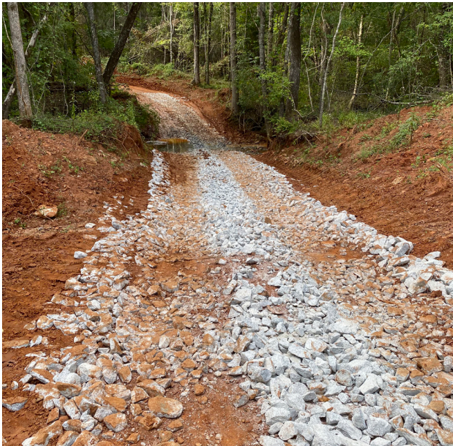
Figure 9. Ford stream crossing. Correct: Use of large rock on forest road and stream crossing during wet-weather harvesting. However, it would be recommended to stabilize the roadsides with straw, hay, or additional rock.
