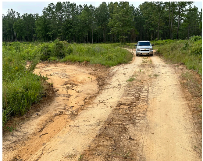
Figure 7. Water diversion device. Correct: Waterbar and turnout installed on a forest road.
