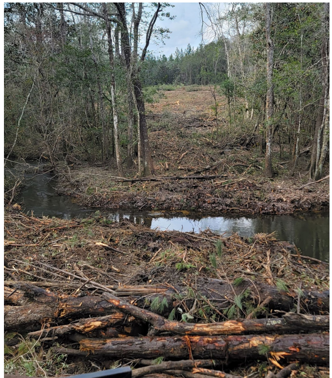
Figure 13. After use, the crossing was removed and the banks were stabilized. (Photo credit: Jason Harrell, PLM Logger).
