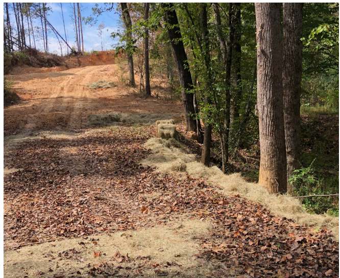
Figure 5. Permanent forest road culvert. Correct: Use of hay or straw on fill slopes and critical areas.
