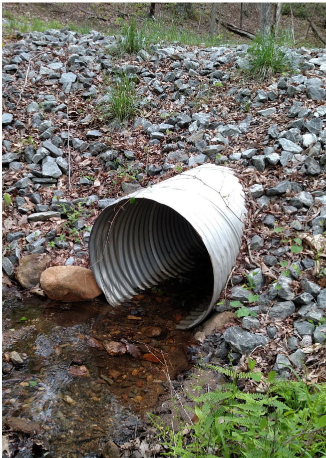
Figure 4. Permanent forest road culvert. Correct: Installed at gradient level for fish and aquatic organism passage and utilizing rip-rap (large rock) to stabilize the fill material.
