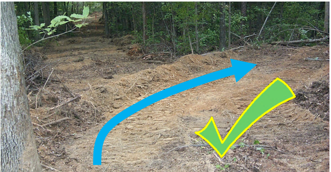
This waterbar ties into a turnout to divert runoff from this closed out skid trail.
