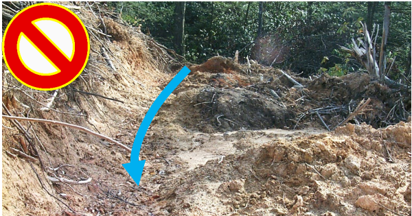
Waterbars are not tied in allowing runoff to bypass around.
