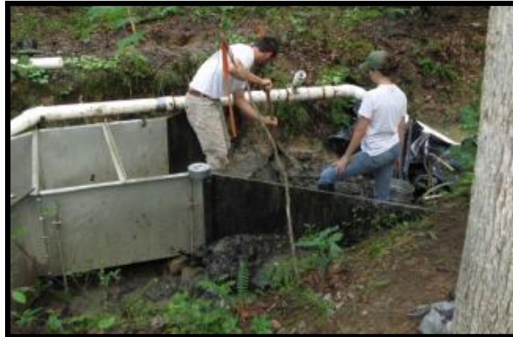
Figure 17. Concrete being added to the entry throat of a flume to keep the streamflow from bypassing under or around.
