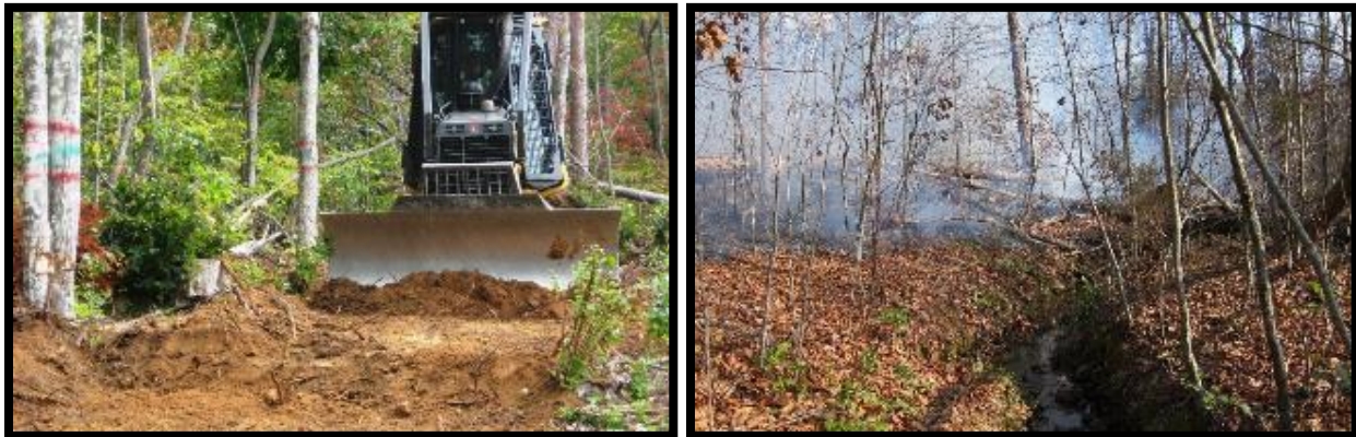
Figure 7. Installation of a fire control line around the perimeter of the UF1 site (right); the operator is installing a waterbar on the fire line. Site prep burn backing out from the Neuse Buffer Rule Zone on the UF1 site
