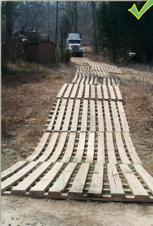
Wooden mats used within the first 100 feet of a public access road can prevent loose sediment from being deposited on the public road surface. While this BMP is designed to reduce nonpoint source pollution runoff, it also helps reduce traffic hazards.
