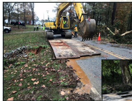
Left: NCFS bridgemats were deployed after flooding washed out an NCDOT roadway in Davidson County.
