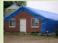
Hurricane Floyd Roof Damage
