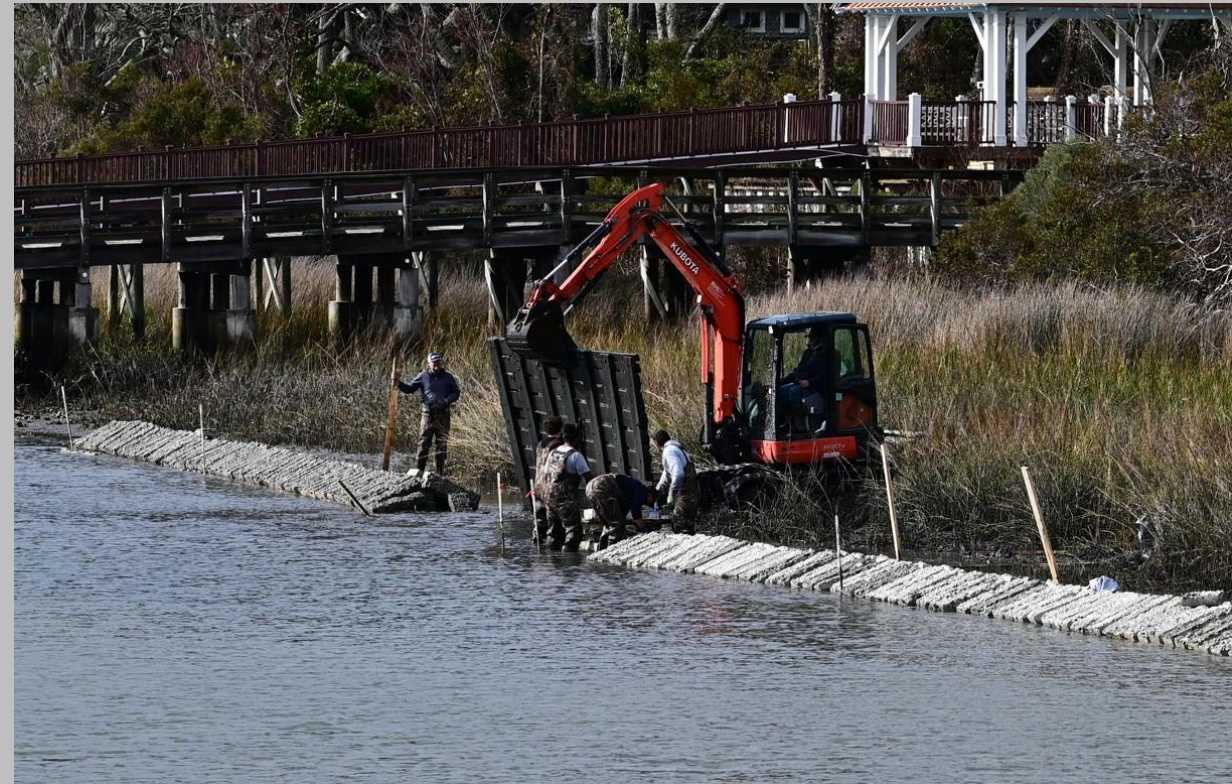
Skid steer removing a mat so the workers can lay the foundation slabs
