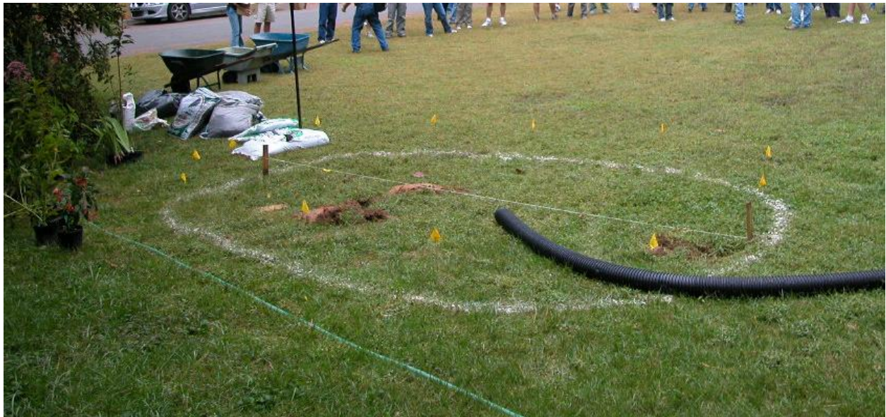
Figure 5.4 Laying out the boundary of a rain garden with paint and flags.
