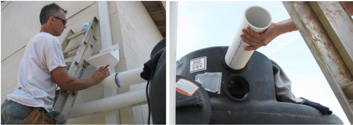
Figure 7.17. (a) Pipe leading from debris filter to the tank; (b) Rubber gasket used to create leak-free seal when pipe enters the tank.
