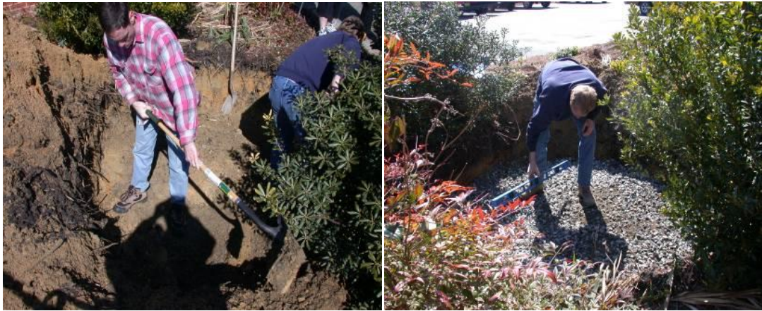
Figures 7.15a Cistern site preparation and b. Preparing the gravel support base.
