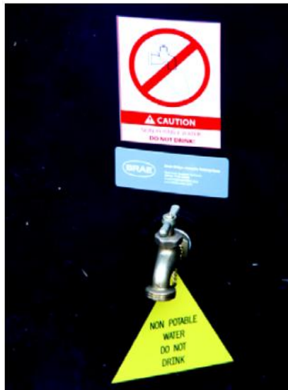
Figure 7.5. Warning signs on a cistern to prevent human consumption of harvested rainwater.
