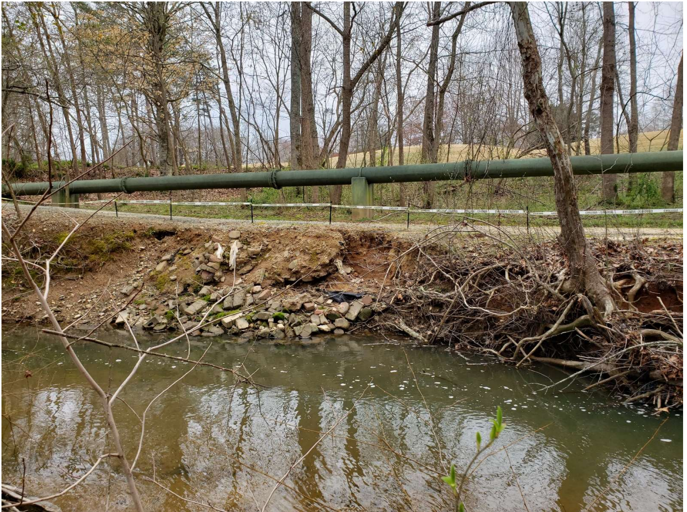
Figure 1: Eroding bank of Rock Creek – March 25, 2021
