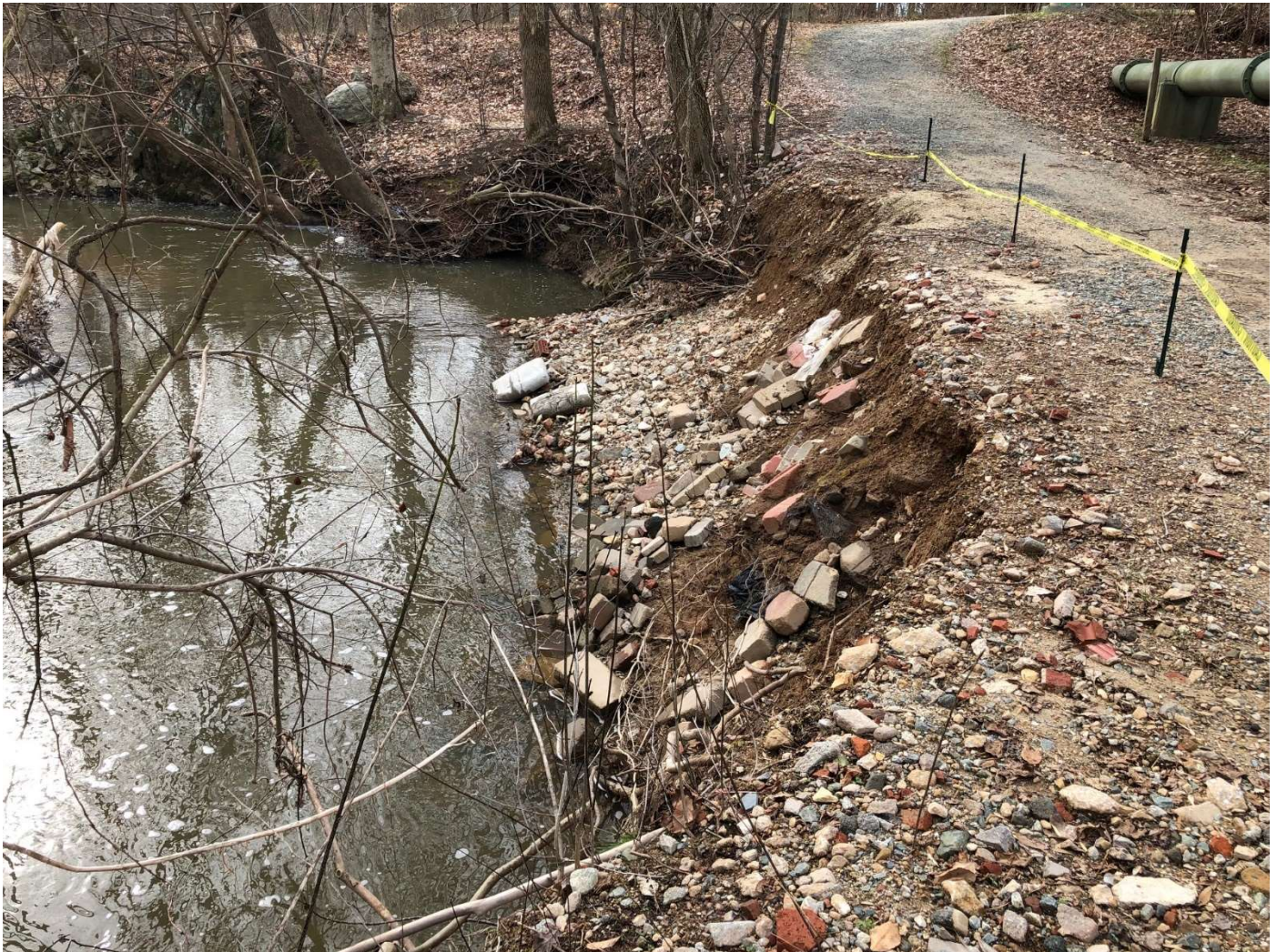
Figure 2: Eroding bank of Rock Creek – January 27, 2019
