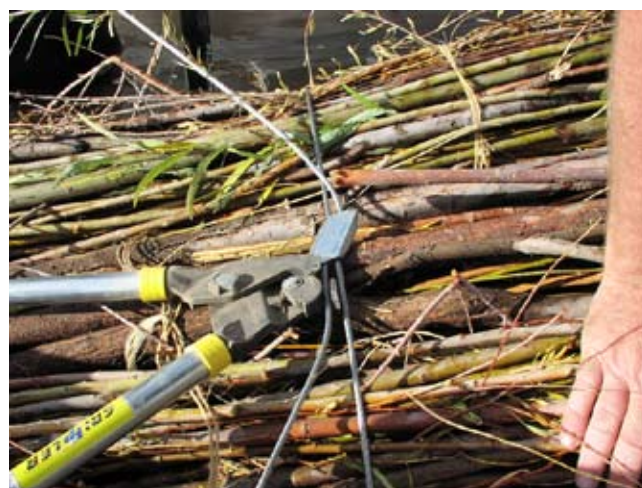
Figure TS14E-12 Gripple® wire rope grip and tensioning tool being used to tension down a brush spur
