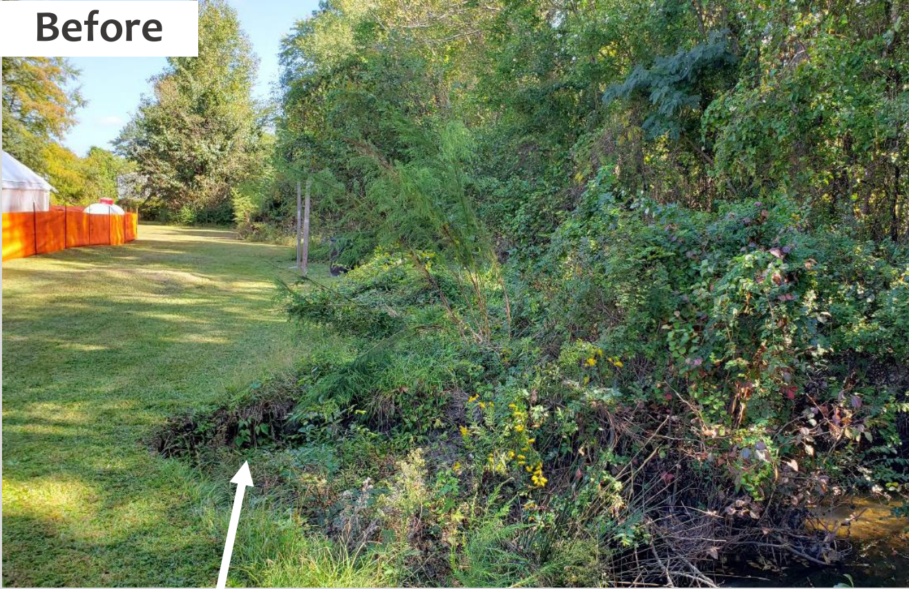
Area of streambank eroding towards building and depositing excess sediment in stream
