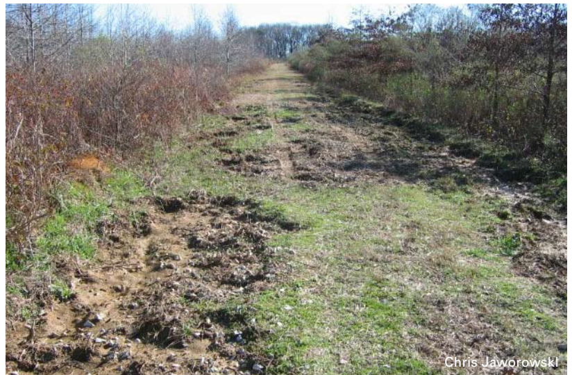
The aggressive rooting tendencies of wild pigs cause damage to roadsides, dikes, and other earthen structures.
